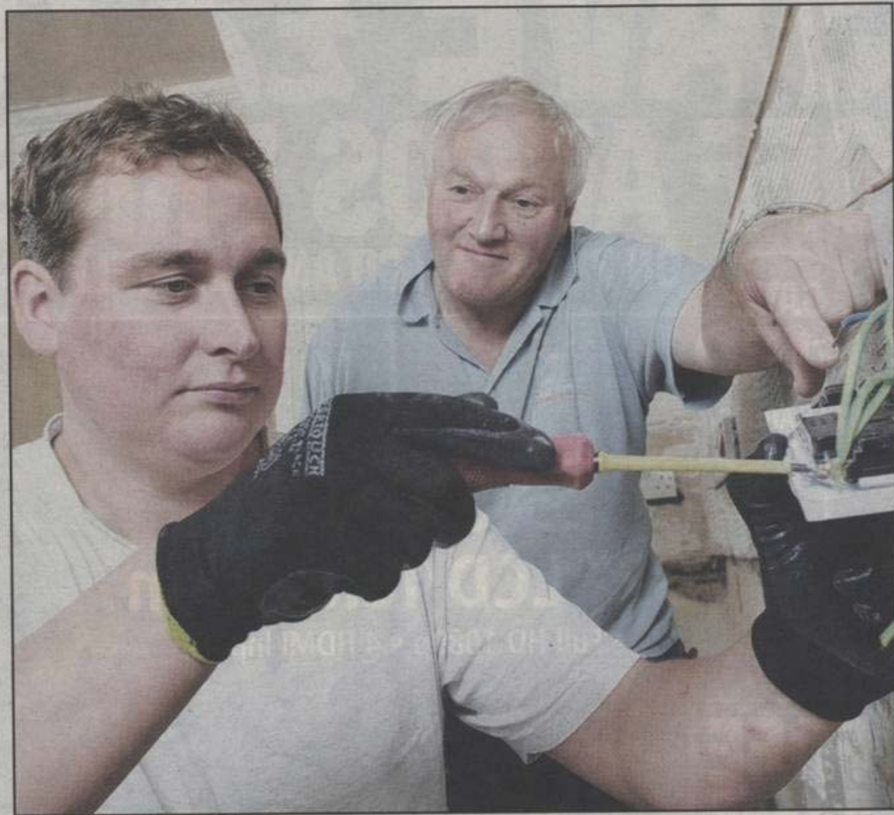
BRIGHT SPARK: Graduate electrician Trevor Capeness (left) learns the tricks of the trade from Walt McMahon of St Leger Homes.
